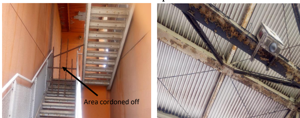
Picture 2: The state of VIP Stand at Accra Sports Stadium at the time of the audit
