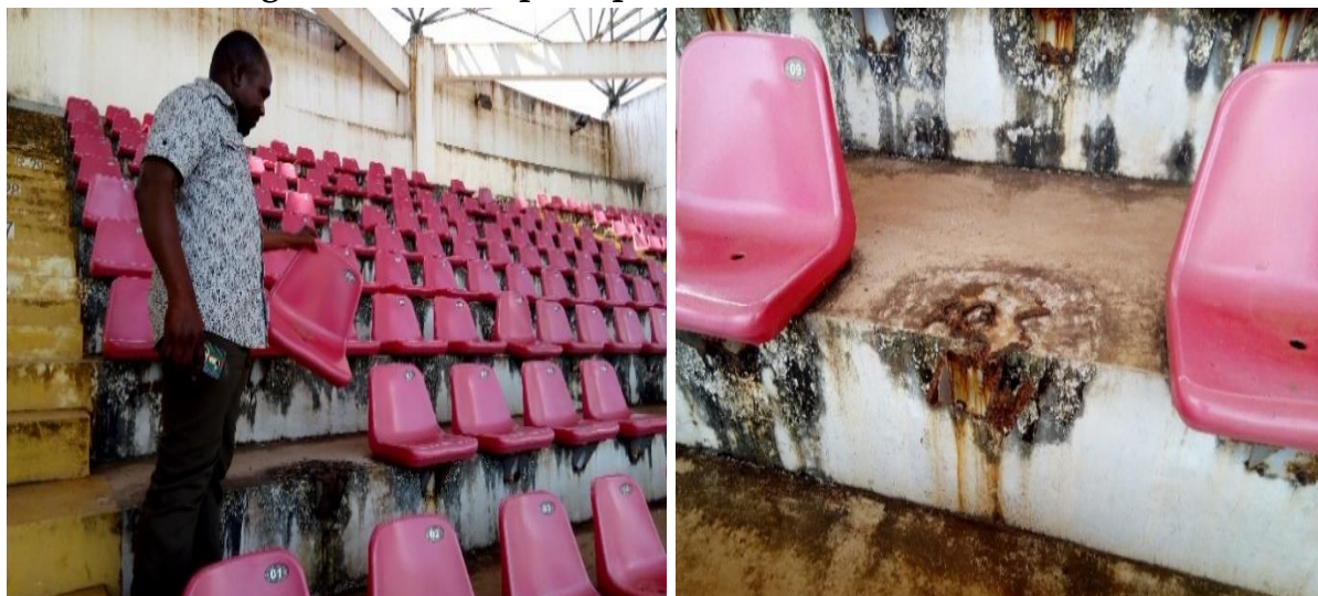
Picture 9: Damaged seats at Essipon Sports Stadium
