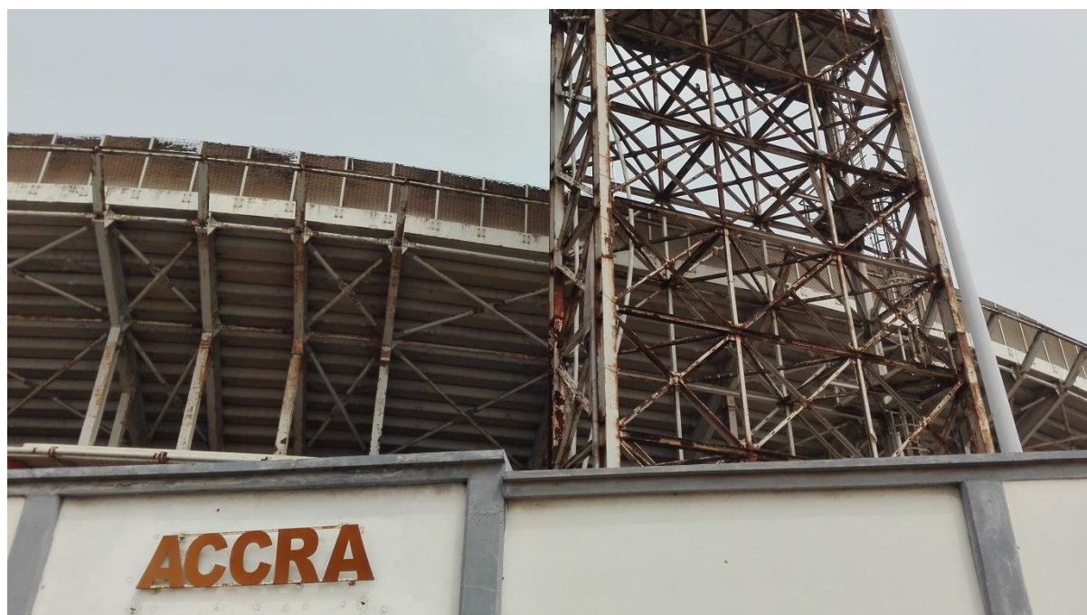
Picture 1: Rusty part of the score board at the Accra Stadium
