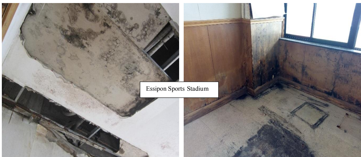
Picture 7: Portions of deteriorated ceiling and wooden wall at Essipon Sports Stadium
