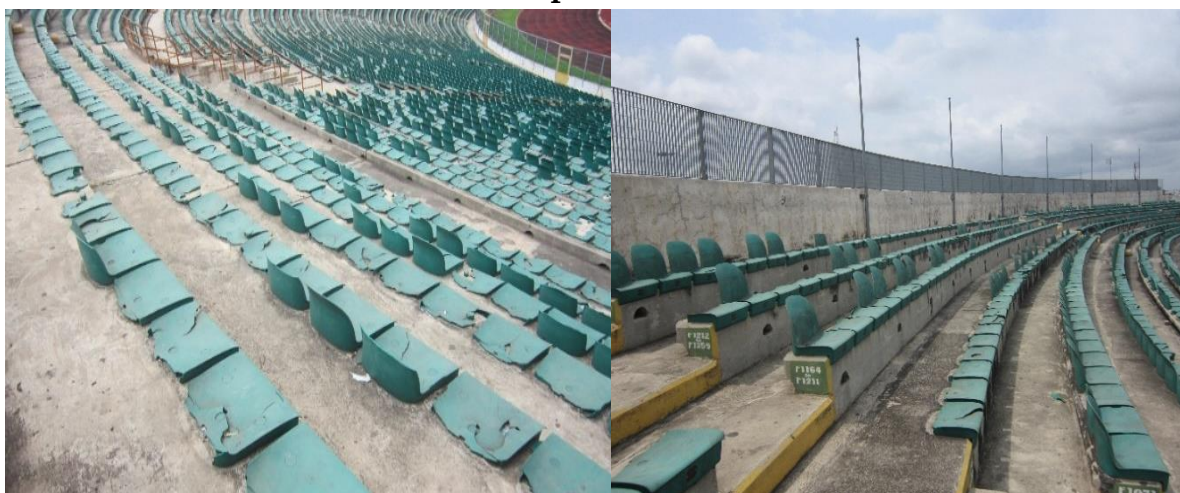
Picture 5: Broken seats at Baba Yara Sport Stadium
